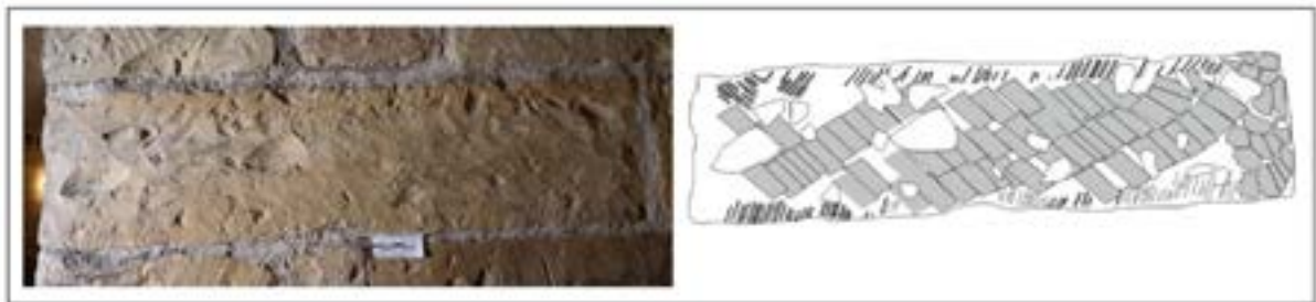
Figure 5. Prague Castle, Basilica of St. George, SE corner of the north arcade wall of the main nave, after 1142 AD. A neat trail cut by the edge of an axe diagonally in rows. Wide notches indicate mutual inclination of block and axe, less than 45°. (M. Cihla)
